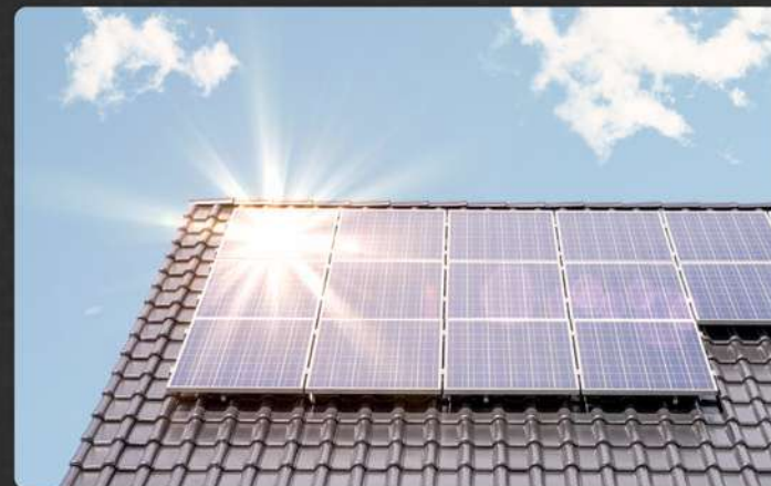
Solar Panel System with Battery
